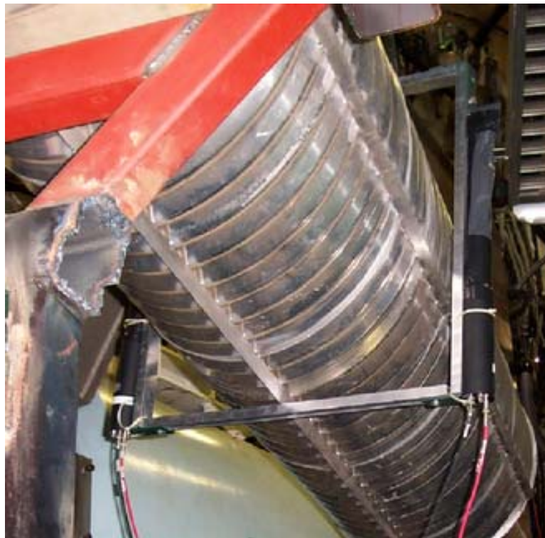
Figure 4: Lumi detector installation around the beam pipe.
