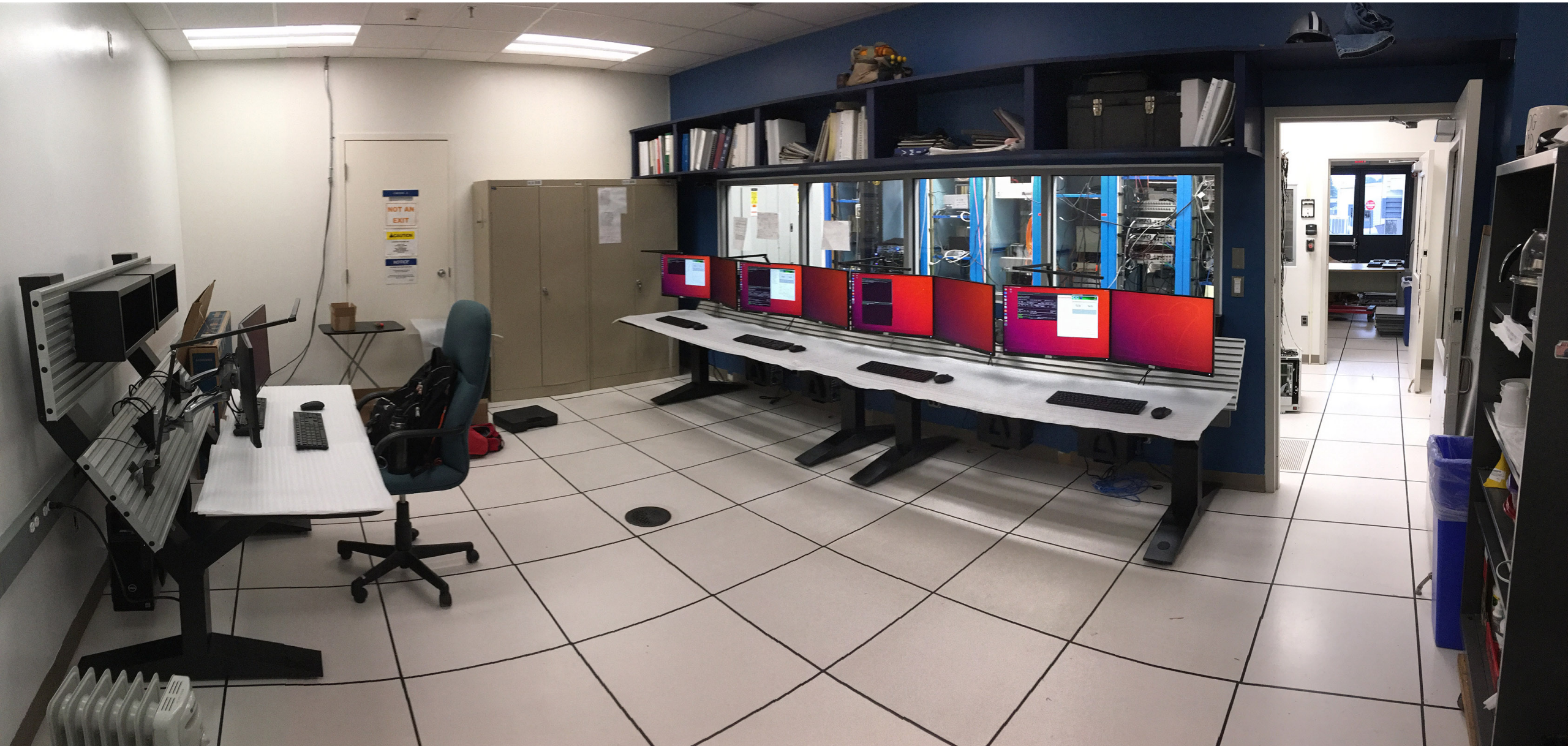
Back room Aug 22, 2021: PCs set up, cabled, not yet networked & configured
