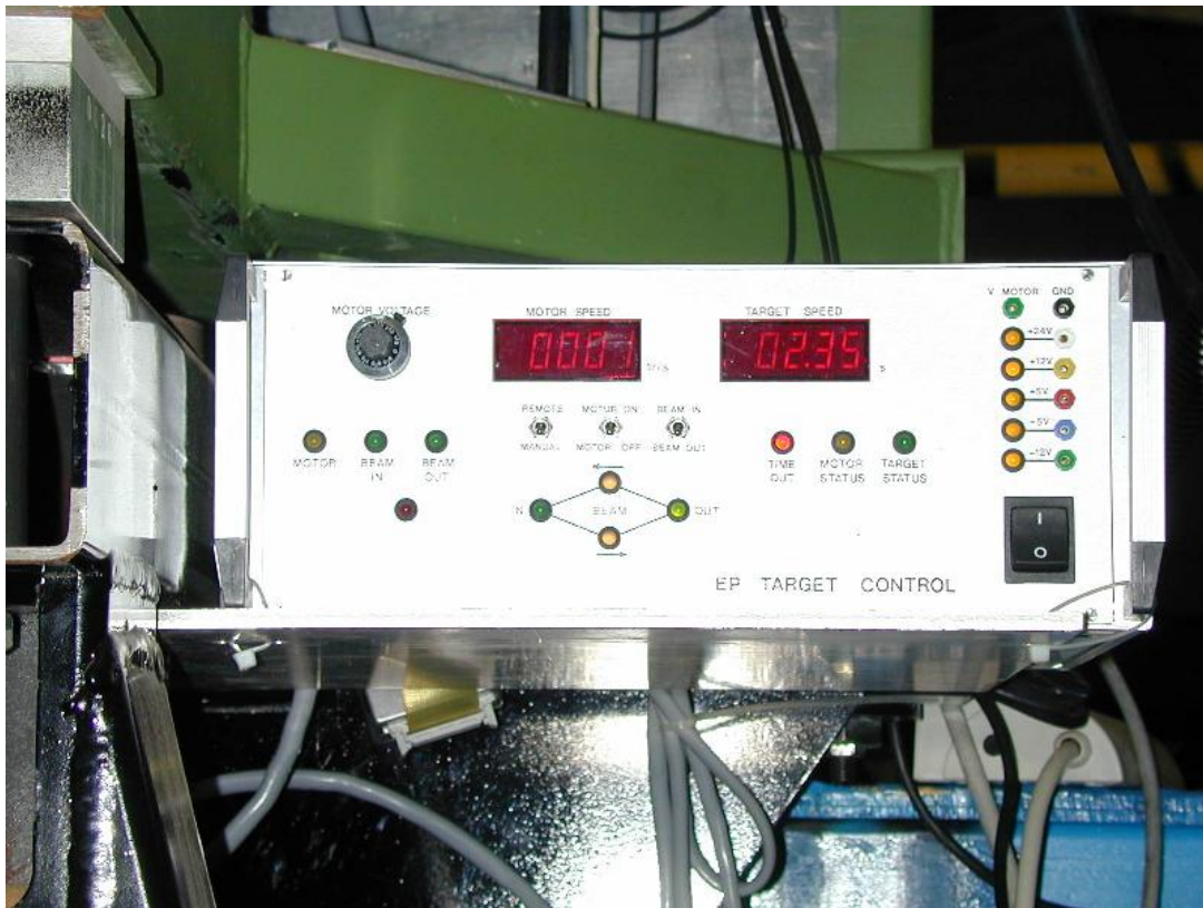
Figure 6.12: Control box for the eP target system.
