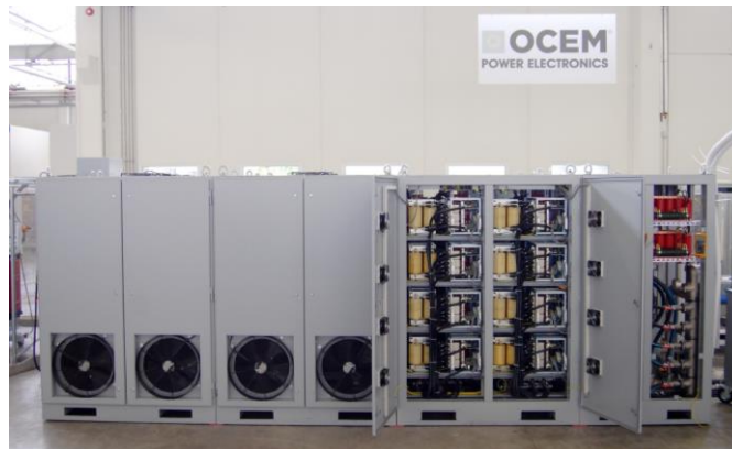
Figure 2 – Example of a complete Power Supply (the picture is related to the TRIUMF Main Cyclotron magnet PS with 8 power modules visible in the front)
