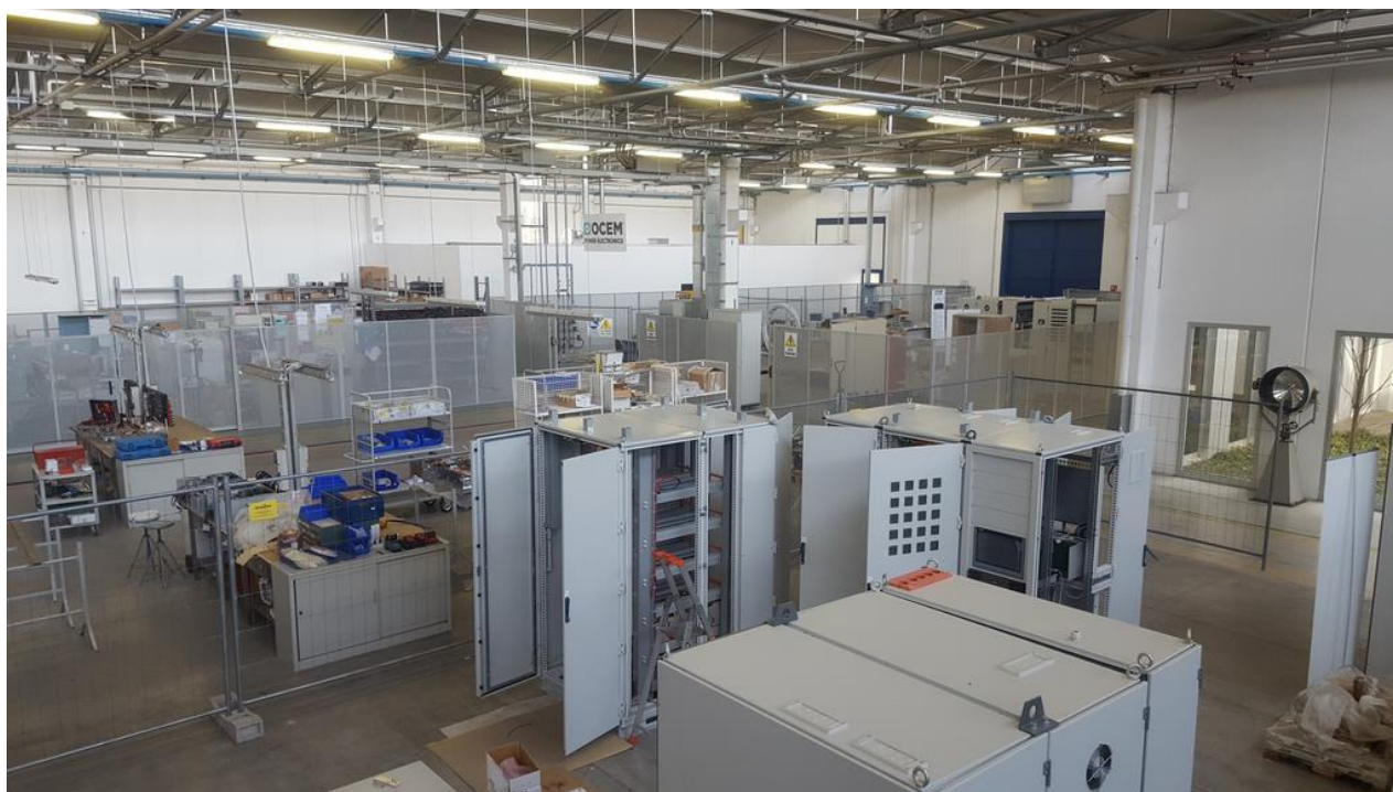
Figure 31: OCEM Production / Test area
