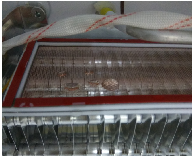
Figure 34. Waterdrop on Surface of Sensor
