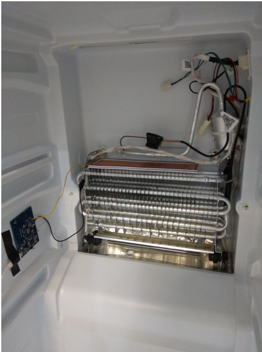
Figure 23. Evaporator In Refrigerator
