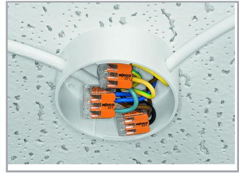
Lighting distribution in a ceiling canopy
