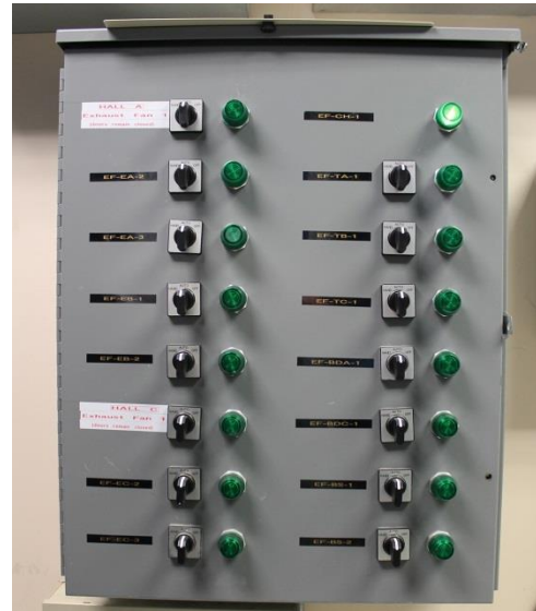
Figure 3. Fan Controls in the MCC
