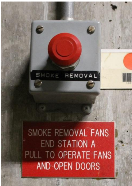
Figure 2. Smoke Removal Button
